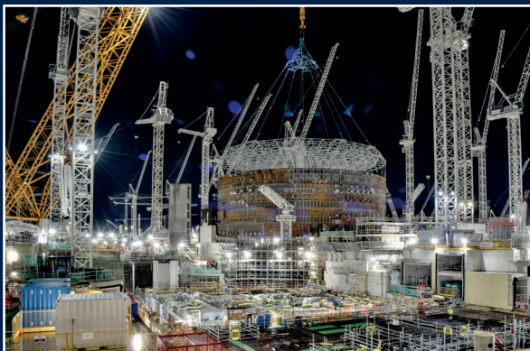
▲ HPC PROJECT PROGRESS INSTALLATION OF THE CONTAINMENT LINER © EDF HINKLEY POINT C MEDIA TEAM
